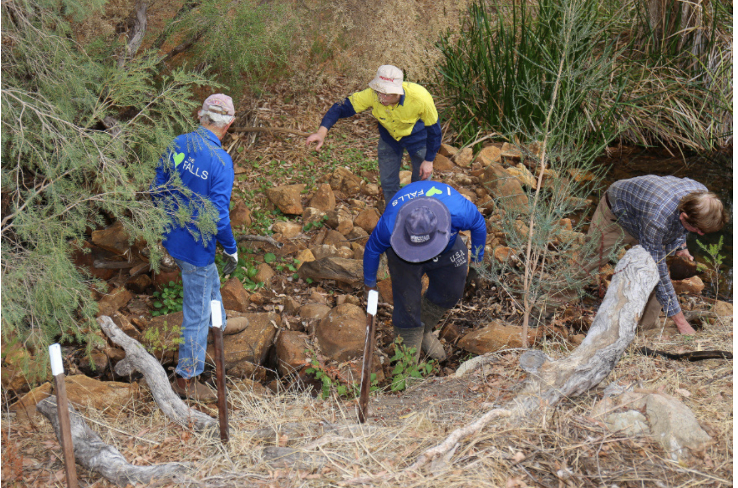
A team used rocks from the creek bed to protect the creek banks and improve flow.
